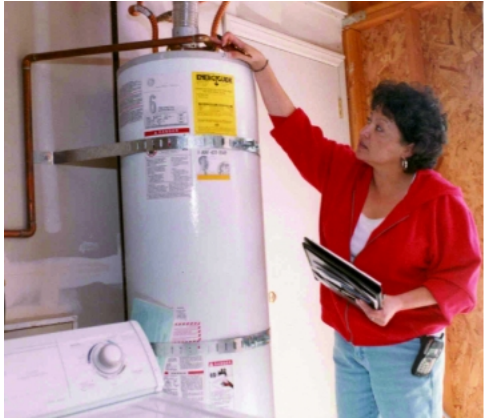
The Housing Commission’s Martha Brownlee makes sure a water heater is properly installed.
